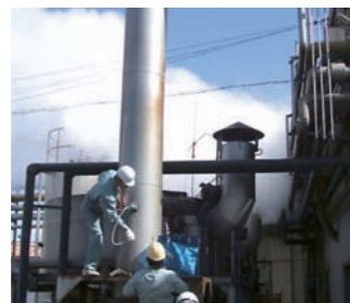
VOC measurement at an exhaust vent
